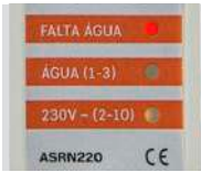
Indication of lack of water in the well (red LED)
